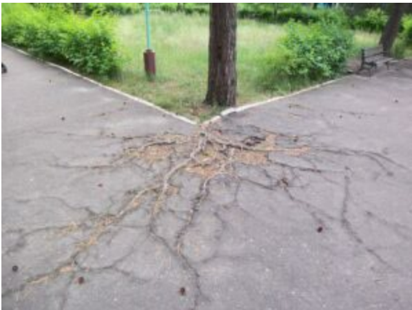
The roots of this tree are demonstrating the destructive power of root wedging. Though this picture is an anthropogenic "rock" (asphalt), it works on natural rock as well.
