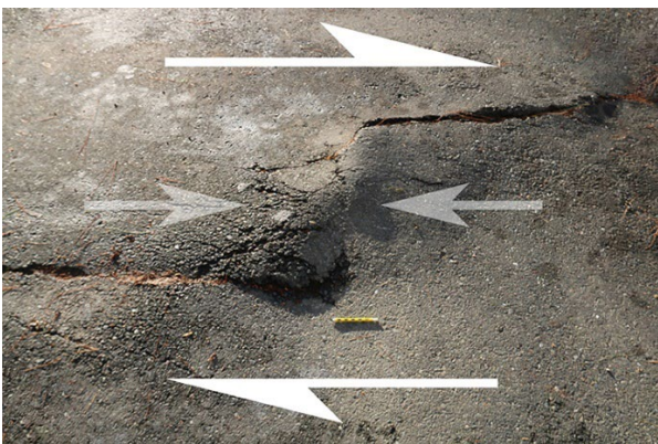
A small pressure ridge developed in parking lot asphalt at Central Park, Fremont, California. This is a left step in the right-lateral Hayward Fault. Perspective is looking to the southwest across the fault.
